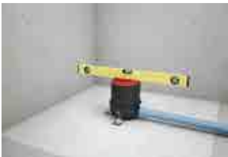
4. Adjust the decline of the pipe by using the angles and level the drain body.
