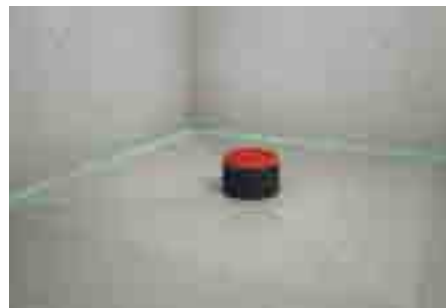
5. Insert floor screed and create a slope to the drain by minimum 2%.
