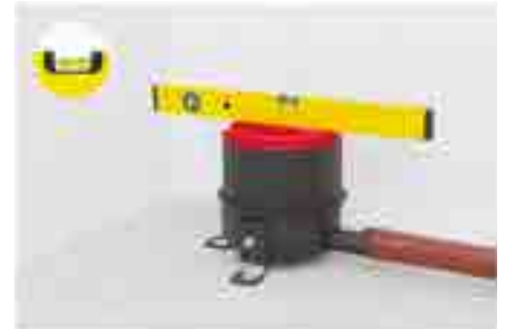
6. Connect drain body with the drain pipe, adjust the slope of the pipe
