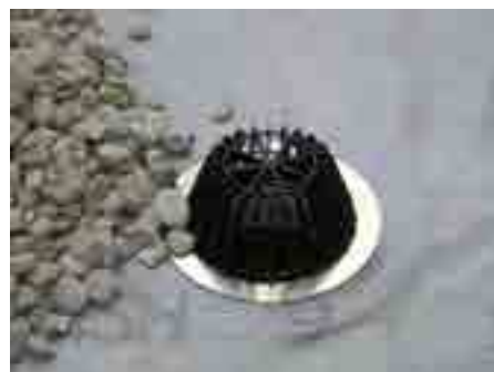
11. Insert leaf catcher, dispense the gravel with minimum grain size 16/32 around the leaf catcher
