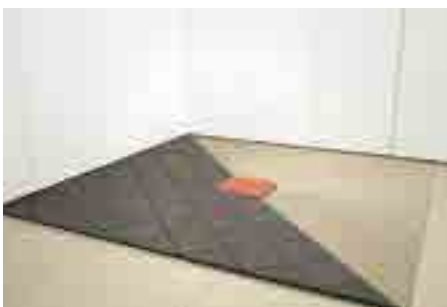
10. Adjust the extension by turning to the tile layout (360° turnable), lay the tiles.
