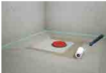
8. Apply waterproofing in the whole shower area and on (and under) the sealing kit, seal the edges with sealing tapes.
